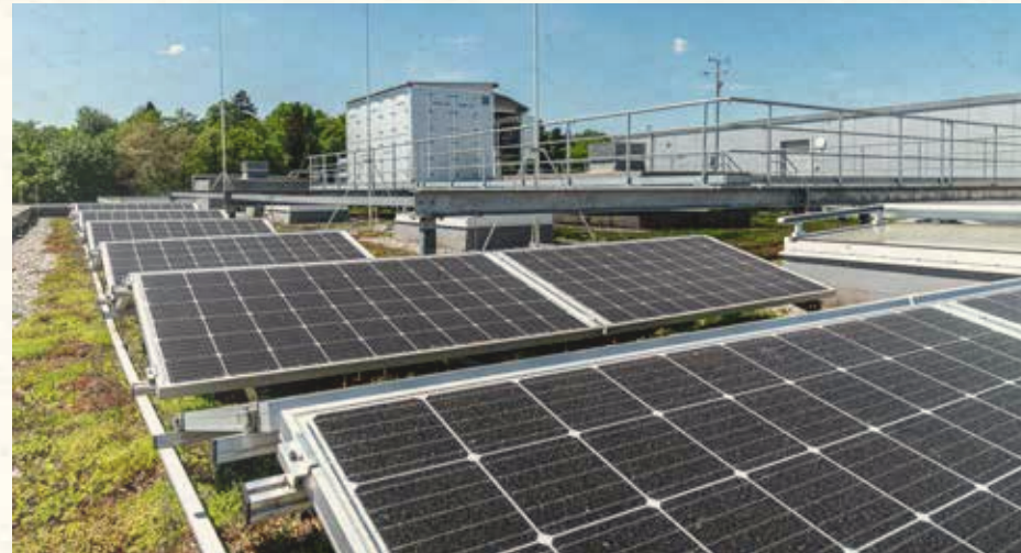
Photovoltaic plant with roof greening at the site Bruckmühl
